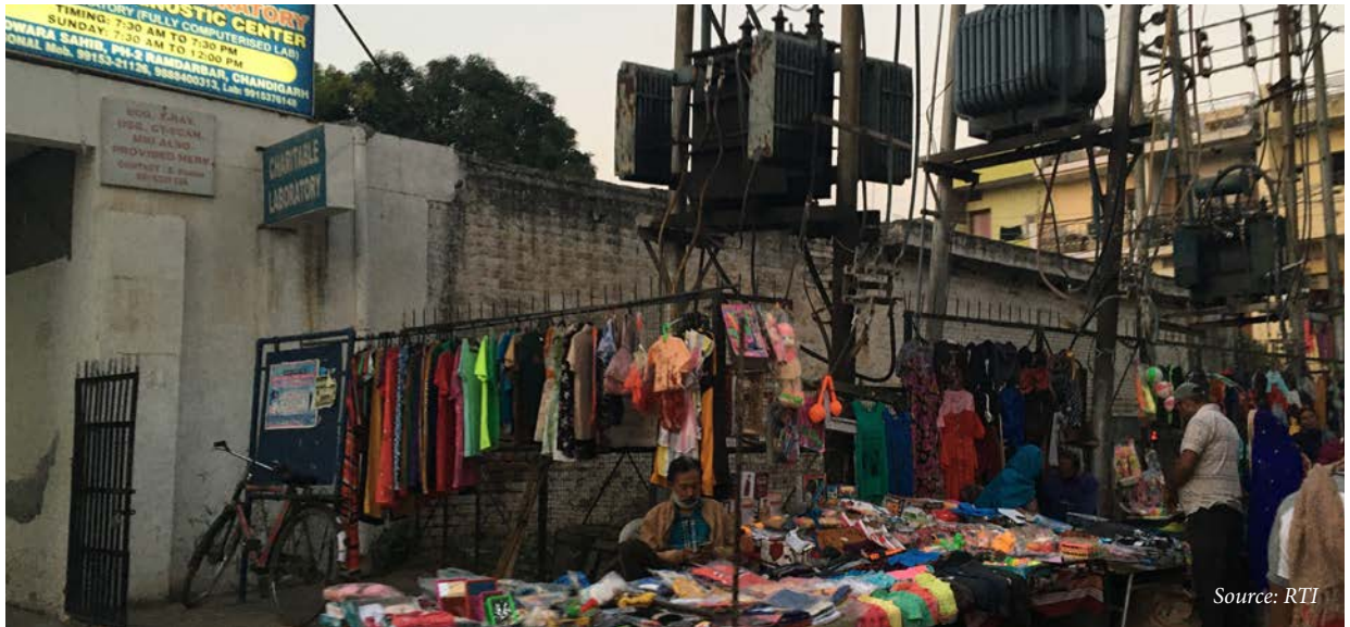
Figure 6.4: Illegal occupancy around the Electrical Transformer (Sector 37)
