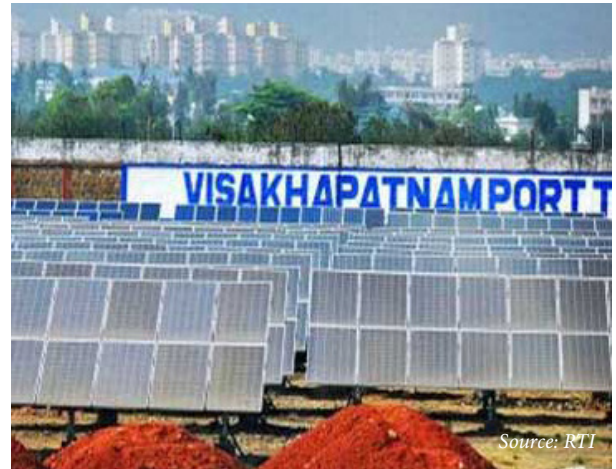
b) Solar Power at Visakhapatnam Port
