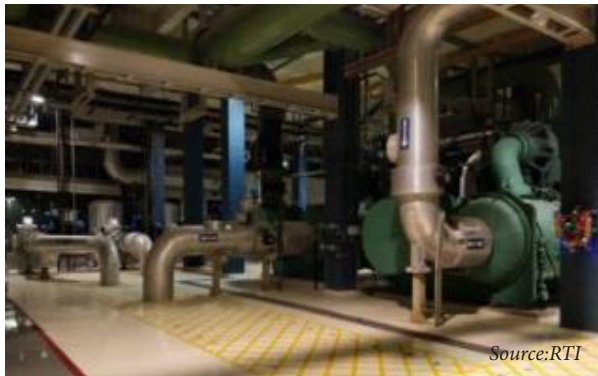
a) District Cooling System
