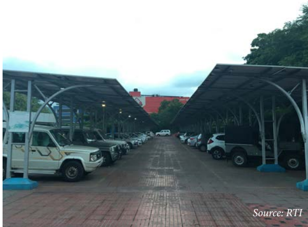
a) Solar Panels installed at GVMC Parking area
