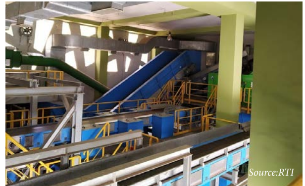
b) Vacuum based Automated Waste Handling System
