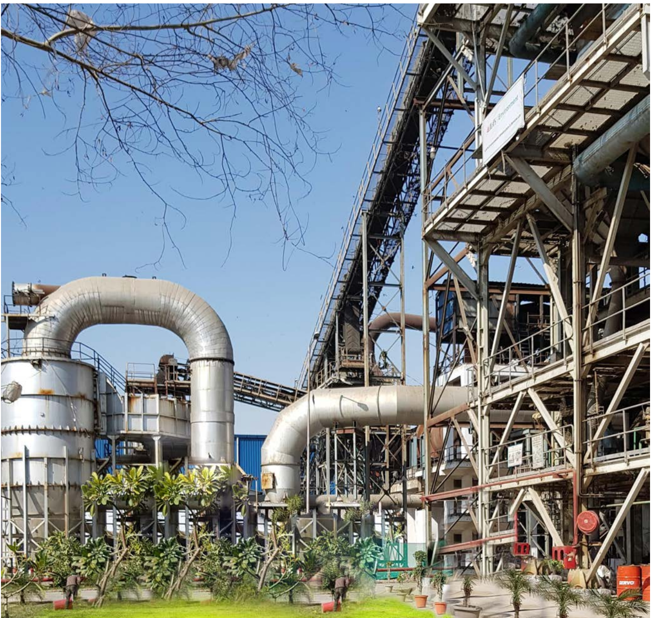
Figure 5.1: Ghazipur WtE plant in Delhi.
